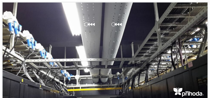
Server room, Leshan City, China
